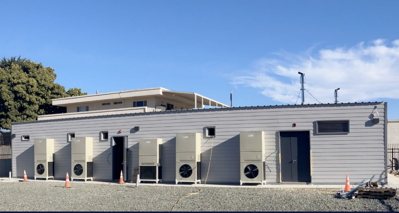
Central Coast, CA cable landing station
